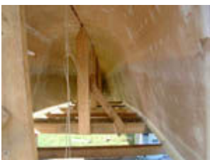
Inside the hull after shaping. Note rudimentary frames, ties, longitudinal grooves in the chine area and transverse dart cuts.
